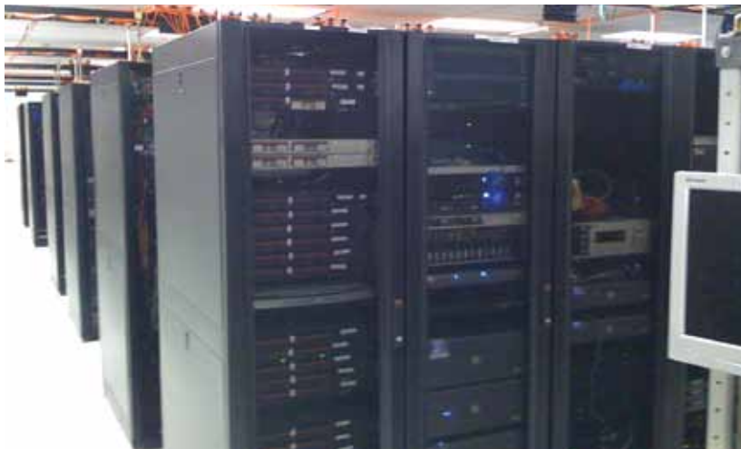
Computer servers connected to the internet.
